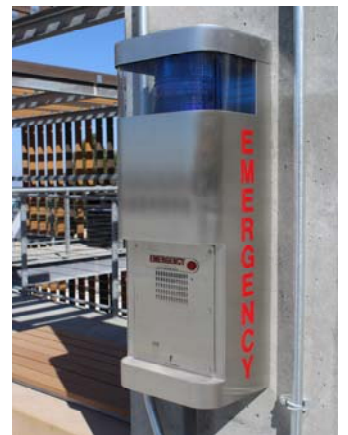
Security Systems Equipment
